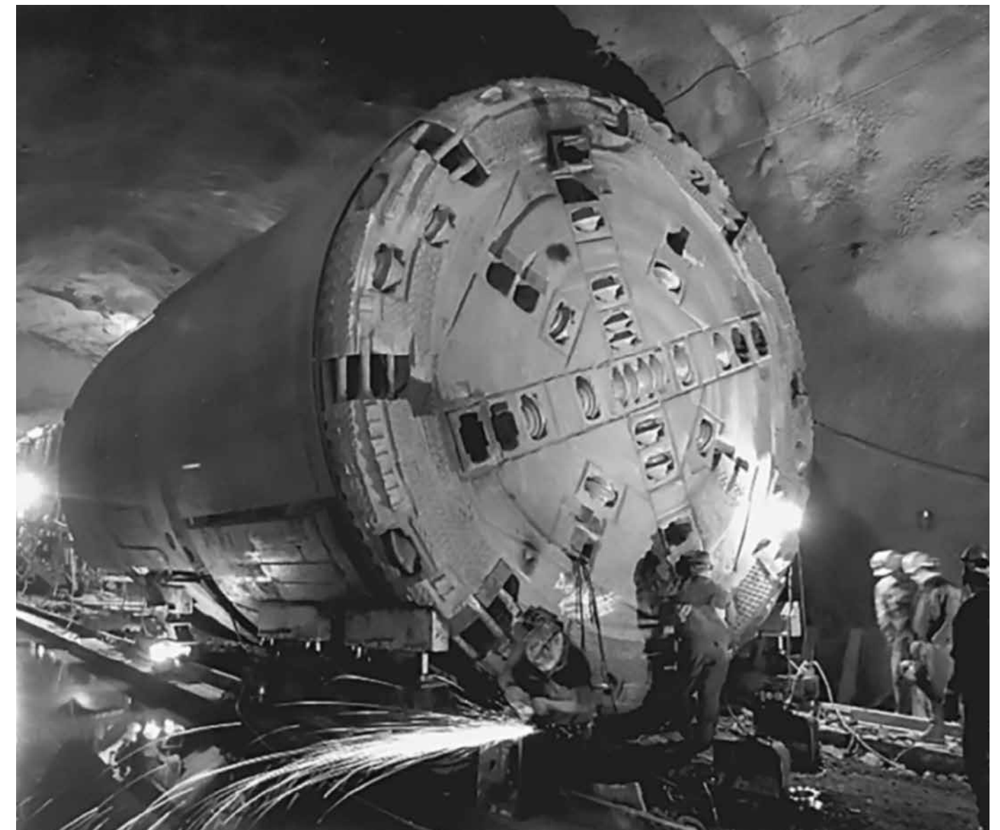
Readying Bore-Regard, the tunnel boring machine, to drill into the west hills during construction of Westside MAX, 1994
